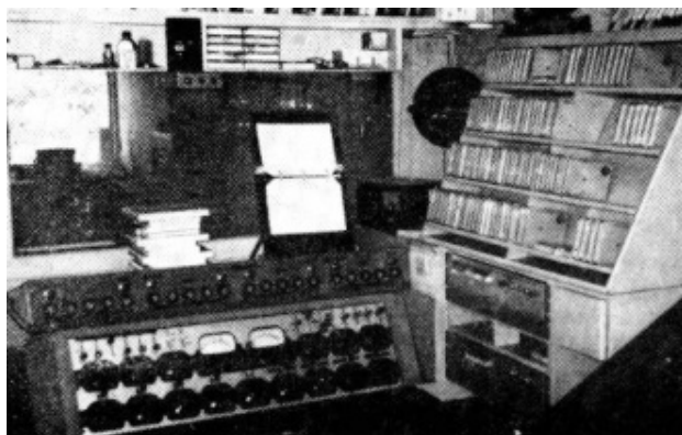
Operating at 1160 kHz on the standard broadcast band, and 6000 kHz on the international broadcast (shortwave) band, Radio Americas routes all program material through control console shown at lower left.
